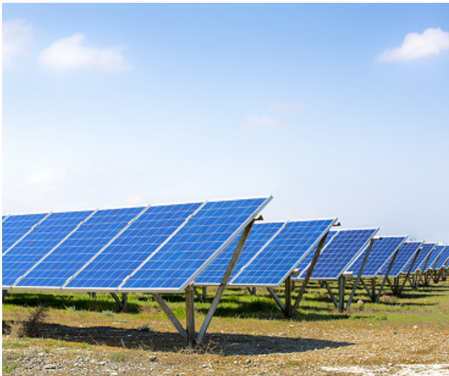
DELTA PLANS TO USE SIMILAR SOLAR PANELS
